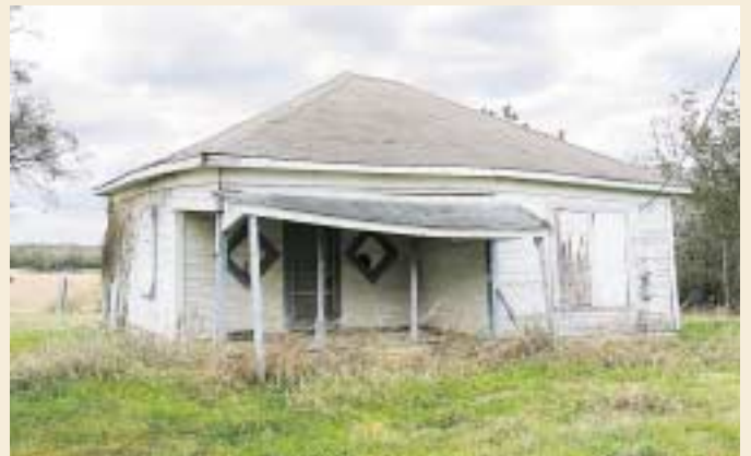
The Rosenwald Fund also helped pay for teachers' homes. This former home is falling rapidly into disrepair.
