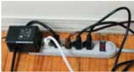
The frequent need for power strips could be a sign that your home's wiring needs updating.
